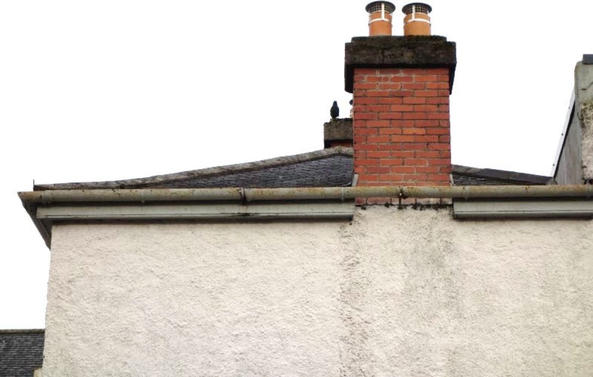
Figure 2: Western side of original building, showing slate tiles and wooden soffit / fascia panels
