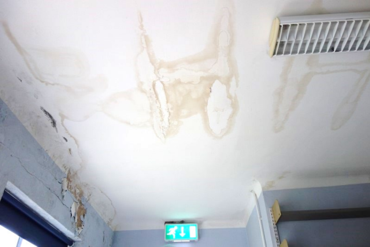
Figure 4: Ceiling damage in upper storey of original building
